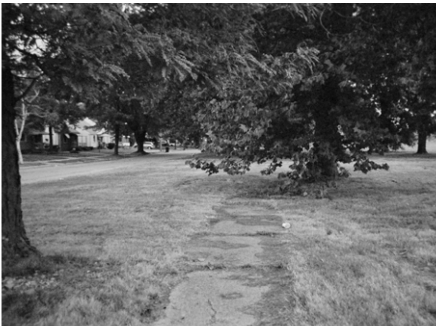
Figure 2 — Broken, overgrown sidewalk.
