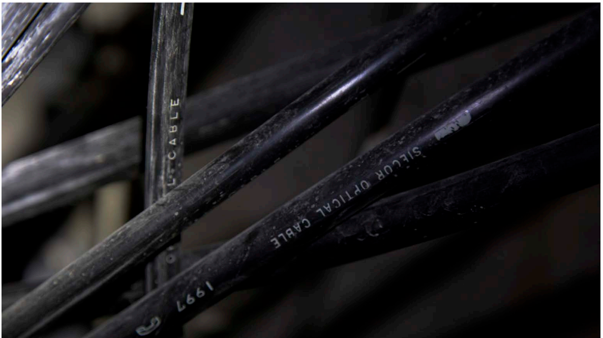
Figure 8. Underground Cable Wires
