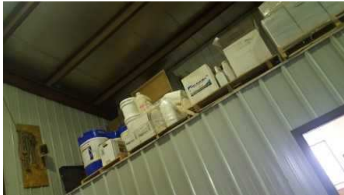
Figure 6. Chemical Storage Above Office
